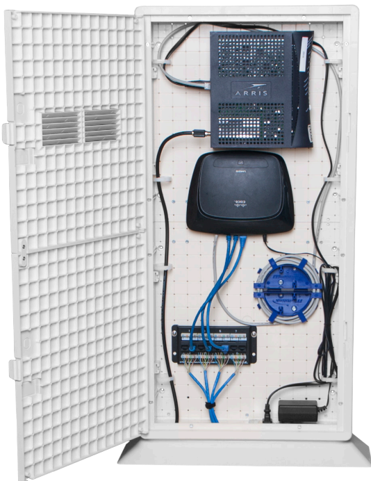
Multi-Media Distribution Enclosure Loaded Example
